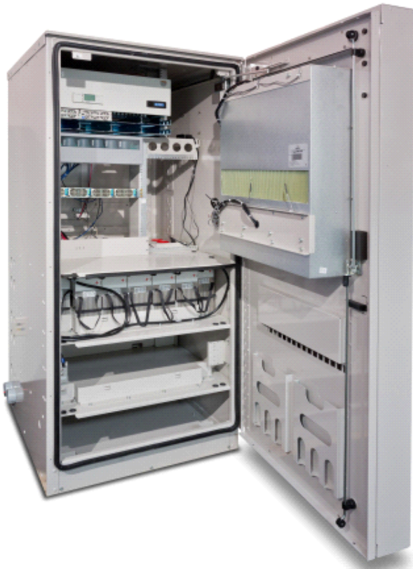
PowerShift is installed at cell sites to automatically deliver the most efficient voltage to remote radio units. (Photo: Business Wire)
