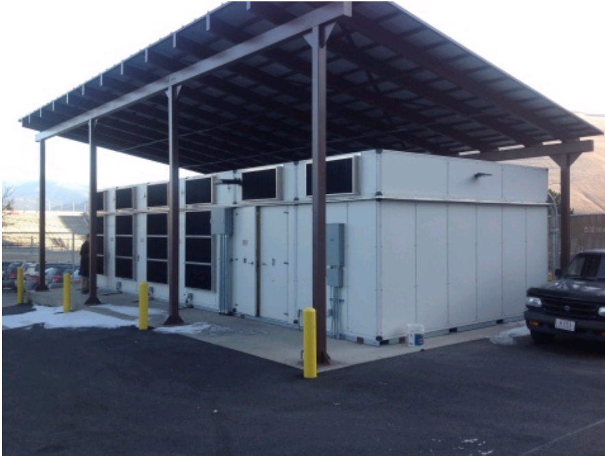
CommScope modular data center at the University of Montana (Photo: Business Wire)
